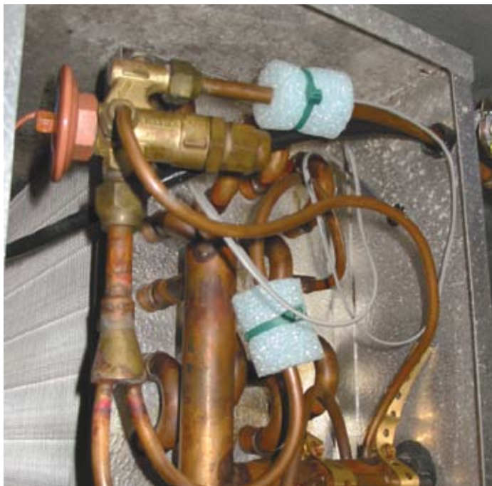
The TDS sensor ends installed on the piping in the evaporator coil.
