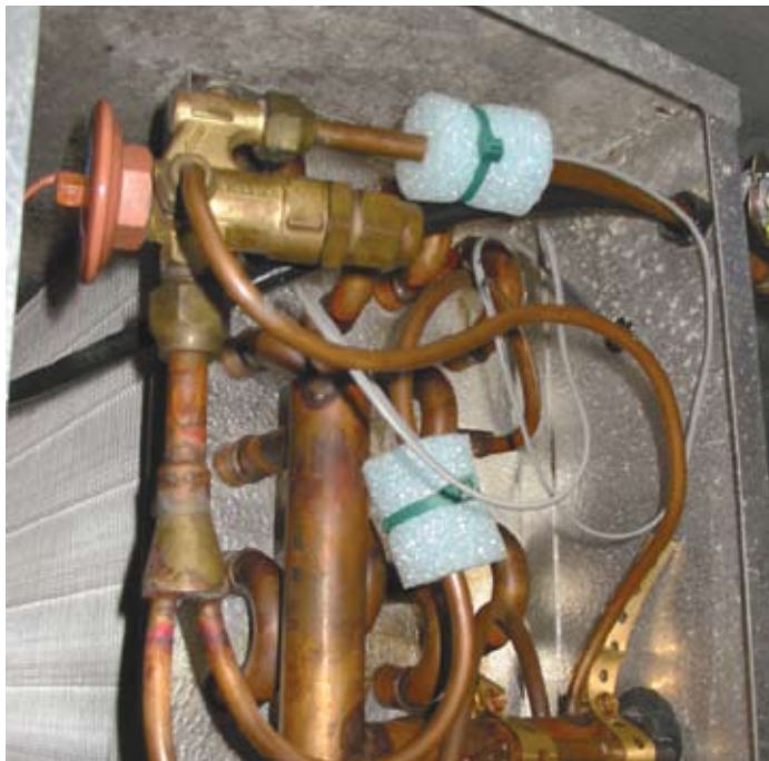
The TDS sensor ends installed on the piping in the evaporator coil.
